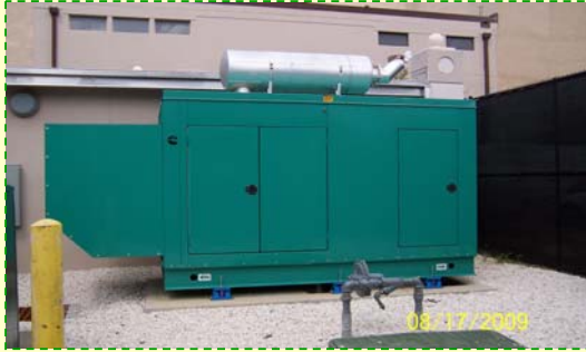
Historic Courthouse County's 1 st natural gas generator – 350 KW
