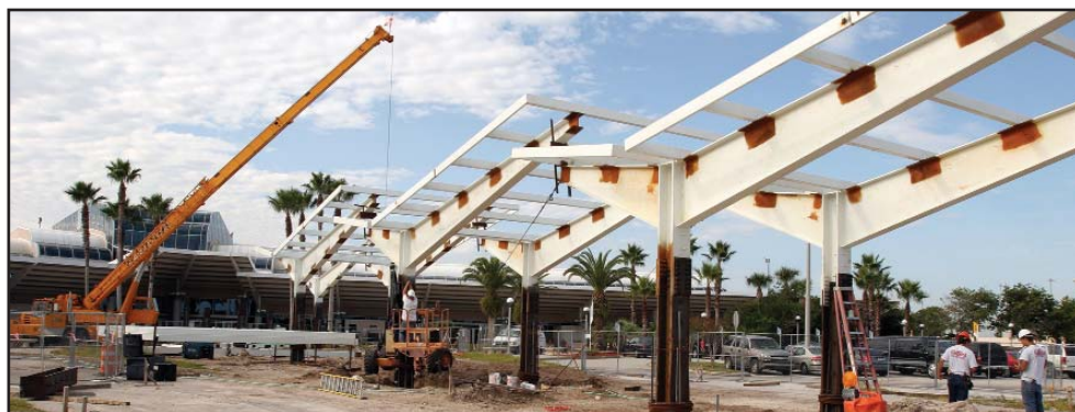
WORK PROGRESSES ON NEW WALKWAY Project will keep travelers safe and dry
