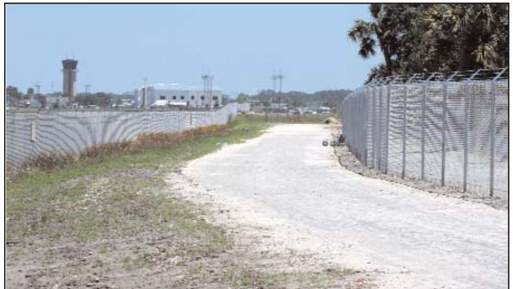
PERIMETER ROAD TAKING SHAPE AT DAYTONA BEACH INTERNATIONAL This is a important safety project that will facilitate the flow of vehicle traffic
