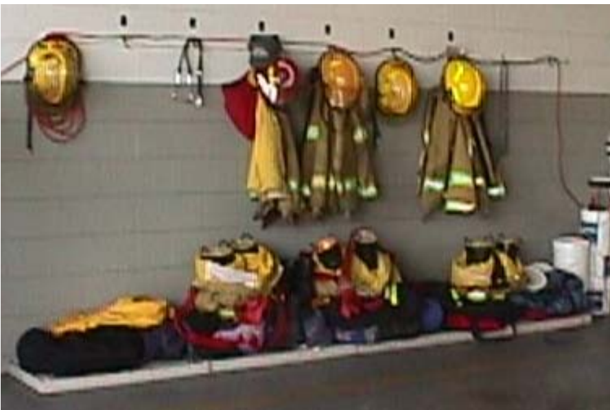
Extension cords plugged into wall outlets and stretched across a wall while being used as a permanent source of power to a battery charger is a safety violation.
