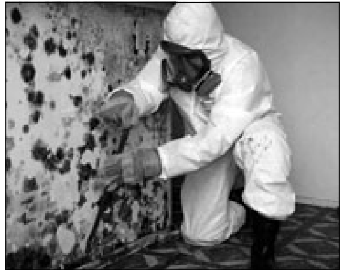
Mold thrives in wet conditions, such as is found following a flood. Here, mold grows on a wall, and a worker is wearing adequate protection for safety. Photo courtesy U.S. Environmental protection Agency.
