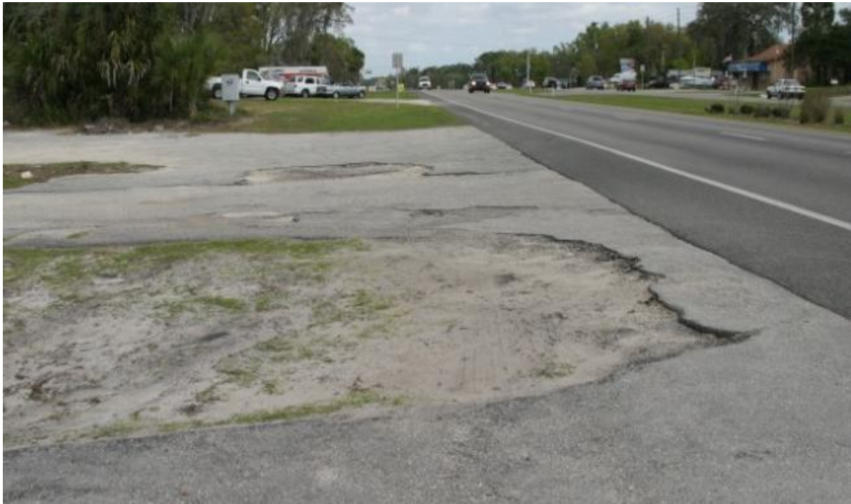
US 17-92 (Volusia Ave.) - Deteriorated driveway
