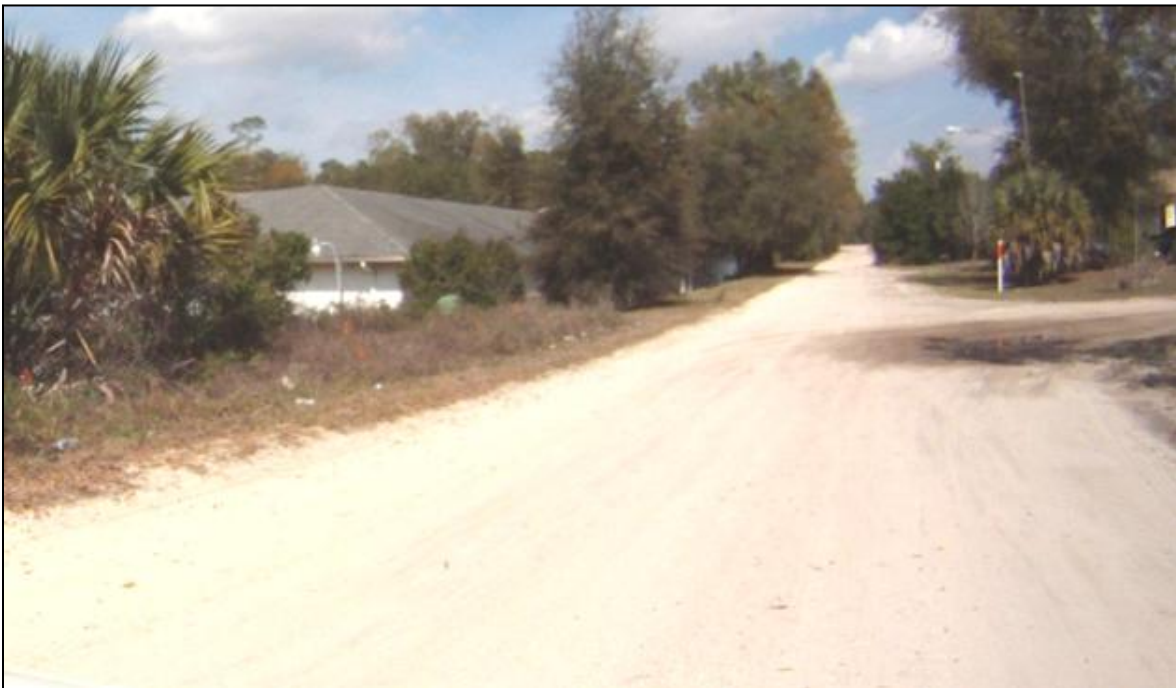
S. Thorpe Avenue. - Gravel road between E. Ohio Ave. to Barbra Ave., poor drainage
