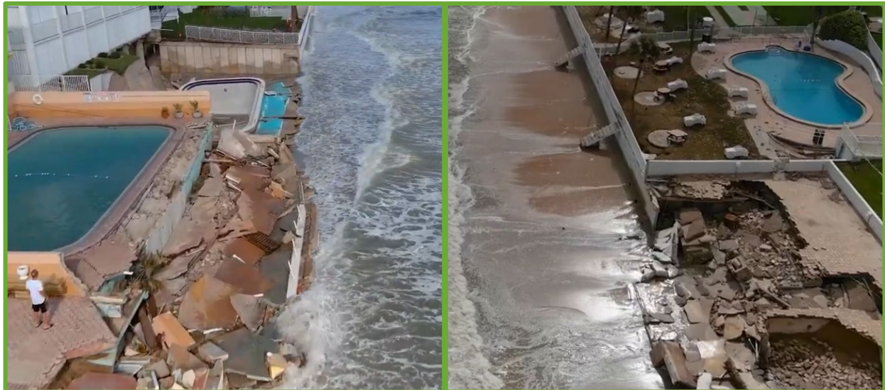
Figure 3: Seawalls collapsed along Volusia County beaches following Hurricane Nicole in November 2022. Since 2022, 29 seawall permits have expired in the County without final inspection. These images illustrate the potential consequences of structural failures in uninspected seawall construction. Source: Volusia County Community Information.
