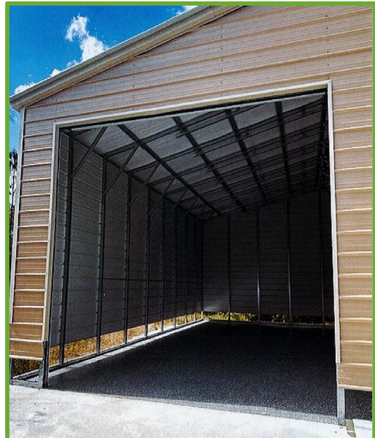
Figure 5: Former Chief Building Official's Workaround for Garage Constructed Below Floodplain
